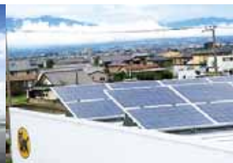
Solar power generation panels
